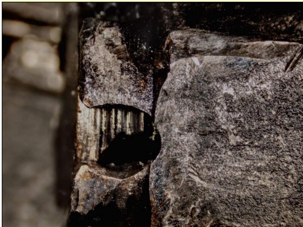
Fig 4 – Female nut on the locking bolt on the connecting rod No.6 is turned and not locked by the cotter pin.
